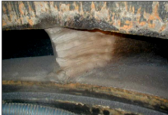
Grit blasted stay vane
